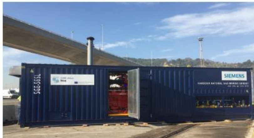
Containerized 56SL genset for harbour use.
