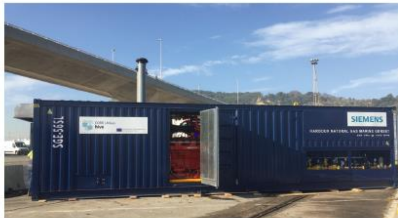
Containerized 56SL genset for harbour use.
